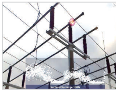
DISCHARGE OF PORCELAIN BUSHINGS ON OUTGOING LINES
