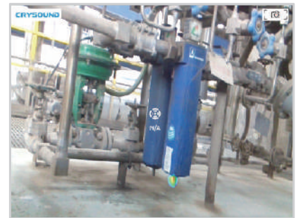
DRY RUNNING GAS SEALS / NITROGEN LEAK
