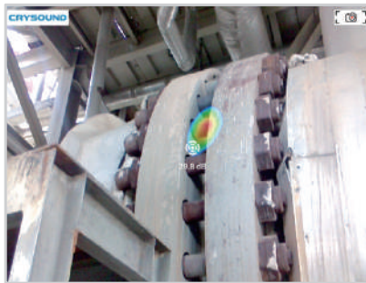
GIANT STEAM FLANGE LEAK
