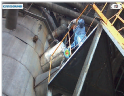
BLAST FURNACE NITROGEN LEAK
