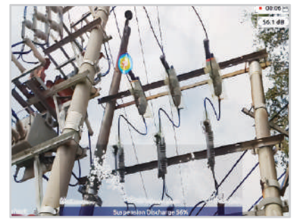
DISCHARGE OF 110KV MAIN BUSBARS
