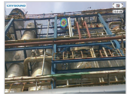
WORKSHOP TOP PIPE JOINT LEAK
